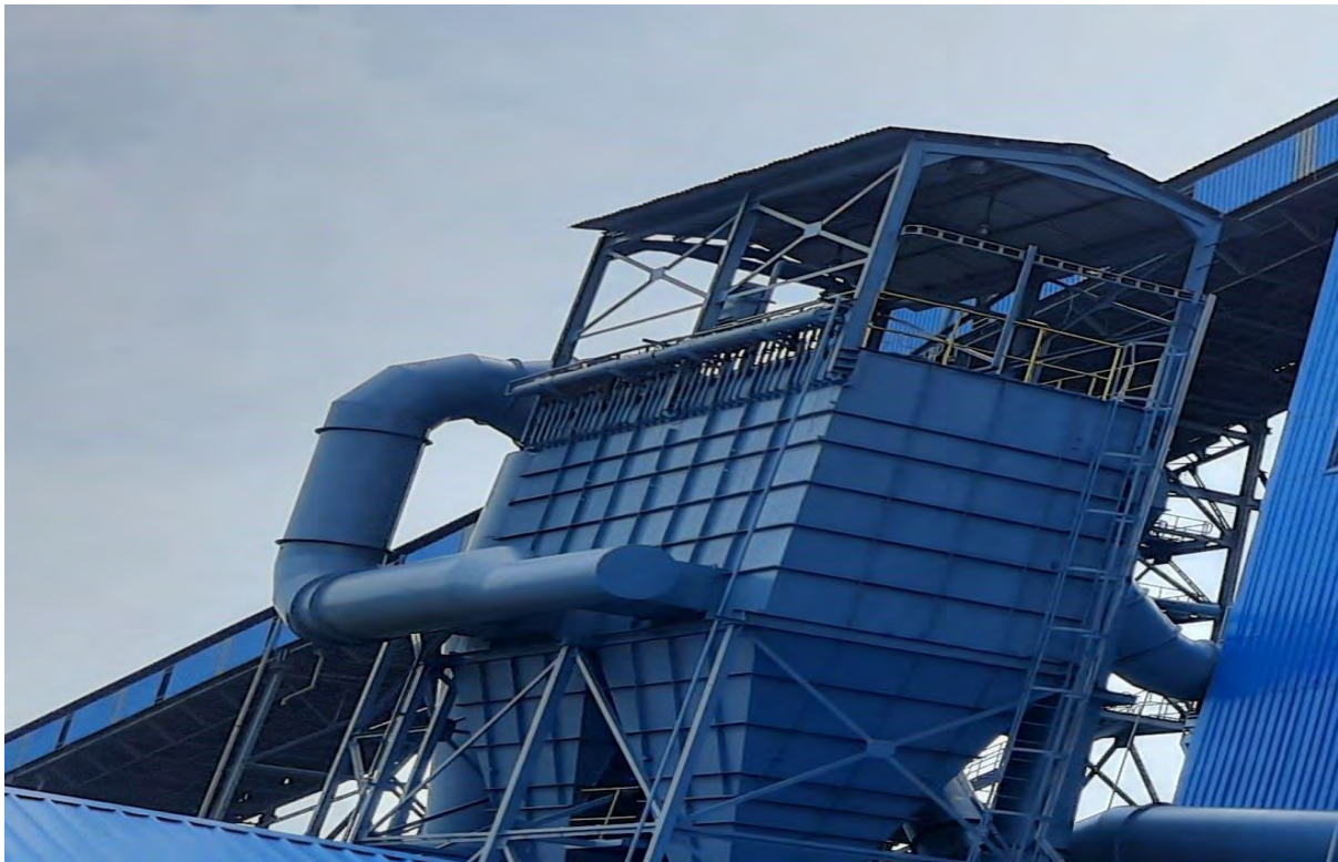
DUST EXTRACTION SYSTEM AT TRANSFER POINTS
